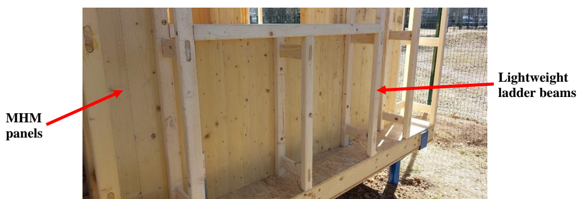
Fig. 1 Solid-wood panels – MHM and lightweight ladder beams in the exterior wall of the research structure.
