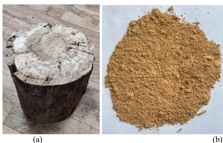
Fig. 1 Rotted wood: a – solid wood; b – disintegrated wood.
